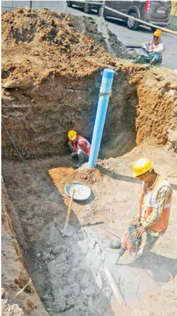
Construction of a few Rainwater Percolation Wells is already being undertaken in the New Campus
